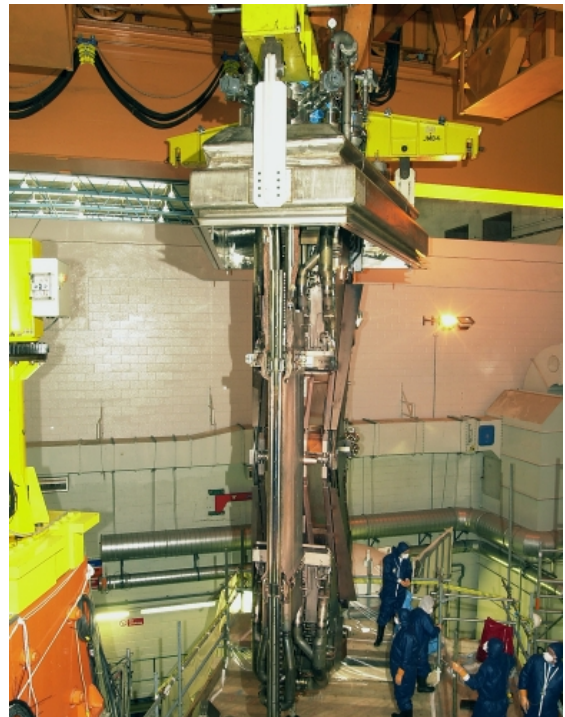
Figure 17: Neutral Beam central column
